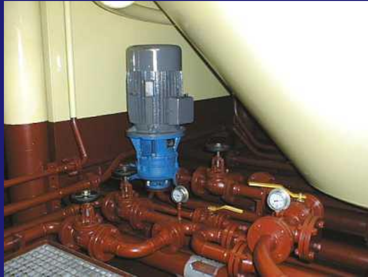
Cleaning pump. (Pumping hot water to the TCM)
