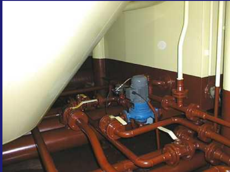
Hot water circulation pump. (Circulating the water between the heater and the hot water tank)
